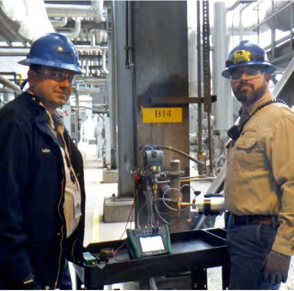
A Maintenance Superintendent, Dustin Ketchem (left) and Combined Cycle Tech, Ron Cash (right).
